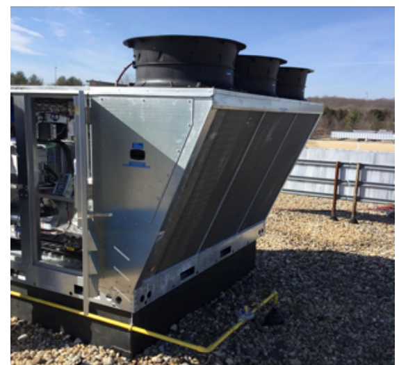
Installed DOAS at the Laboratory
